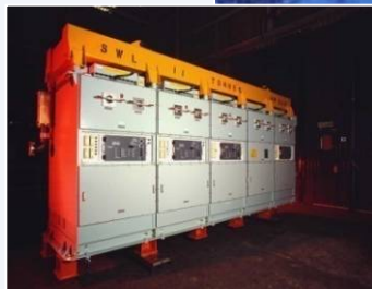
Main static converter
